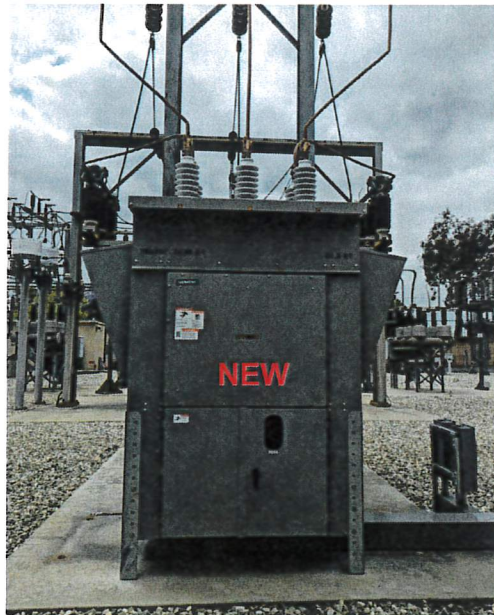
New 34kV Vacuum Circuit Breaker at Valley Transf. Bk. A-1
