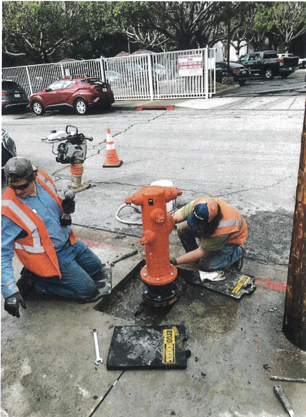
The new hydrant, above, uses the newest technology available and has connections compatible with the latest fire department standards.
