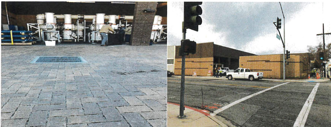
View of 69 kV Switchgear (Left) and Ontario Exterior View (Right)
