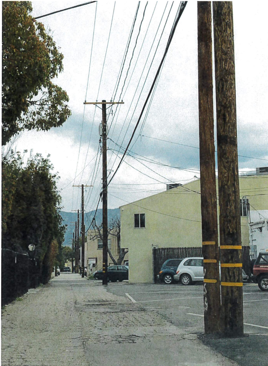
N-21 Alley – 12kV single- and three-phase primary service
