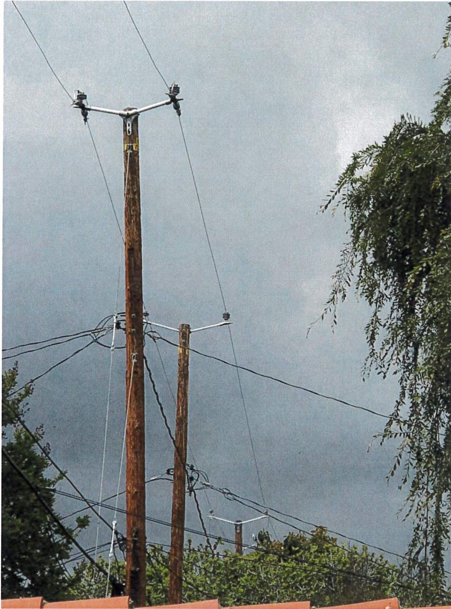
N-21 Property Line – 12kV single-phase primary service
