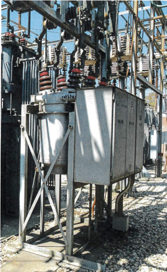
Original 4 kV OCB
