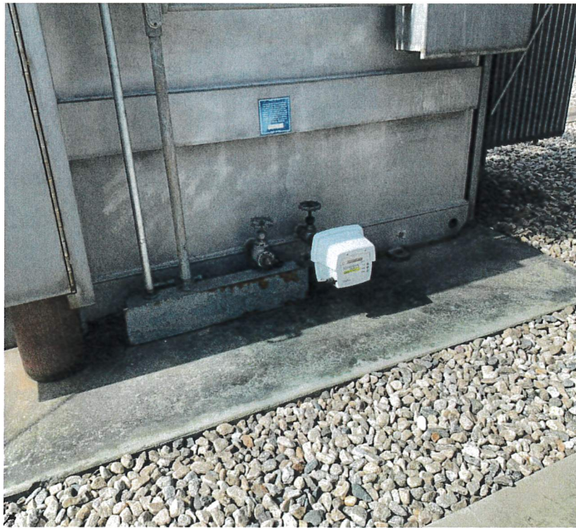
Winona Transformer Bank A-3 Gas Monitor
