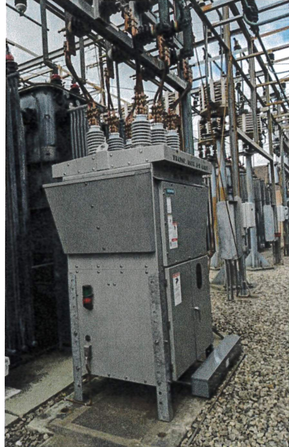
New 4kV VCB
