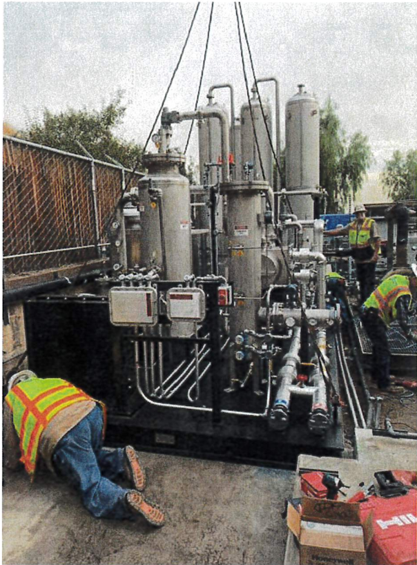
LFG Conditioning Skid
