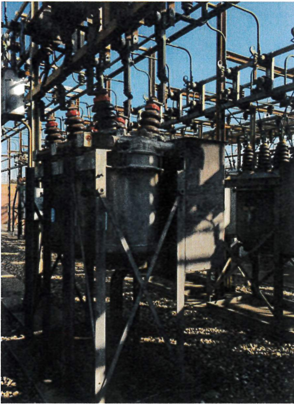
Original 4 kV Oil Circuit Breaker for Flower A-2
