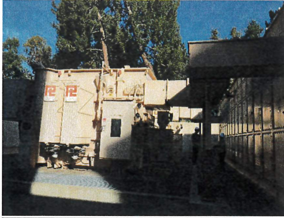
Transformer Bank A-2 Before Installation
