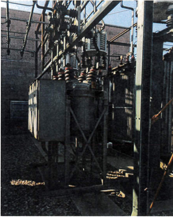
Original 4 kV Oil Circuit Breaker for Flower A-1
