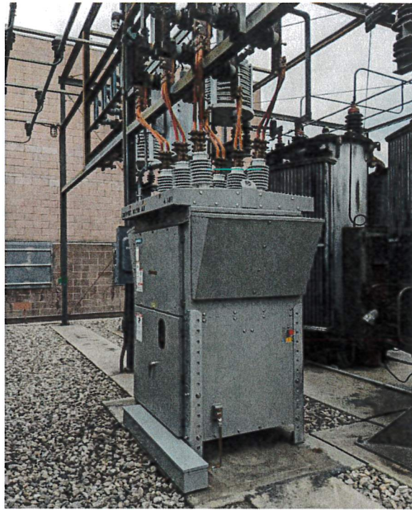
New 4 kV Vacuum Circuit Breaker for Flower A-1
