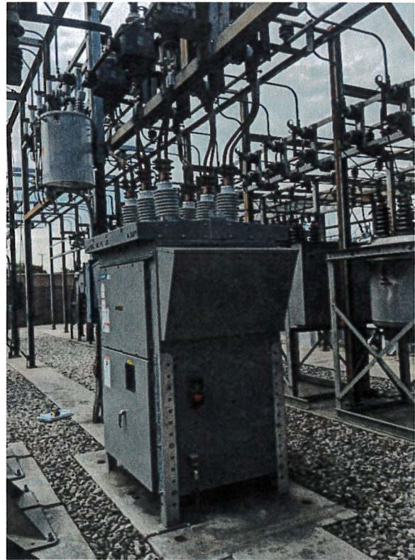
New 4 kV Vacuum Circuit Breaker for Flower A-2
