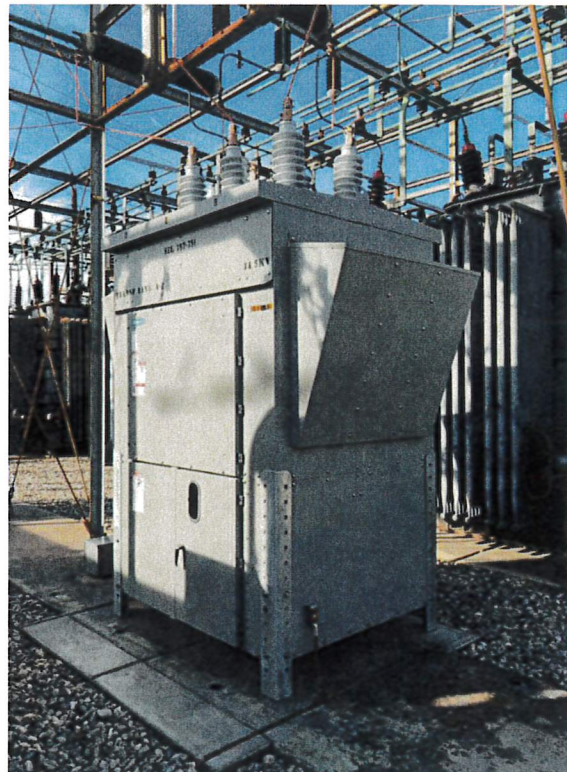
New 34.5 kV Vacuum Circuit Breaker for Winona A-2
