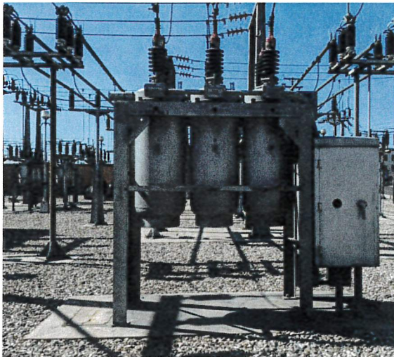
Original 34.5 kV Oil Circuit Breaker for Valley Bus-Tie
