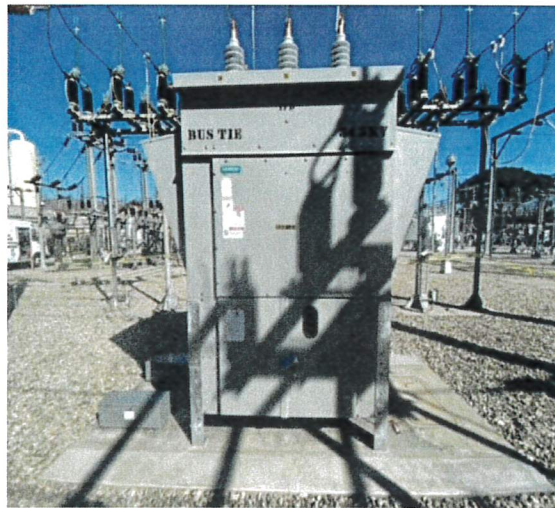
New 34.5 kV Vacuum Circuit Breaker for Valley Bus-Tie
