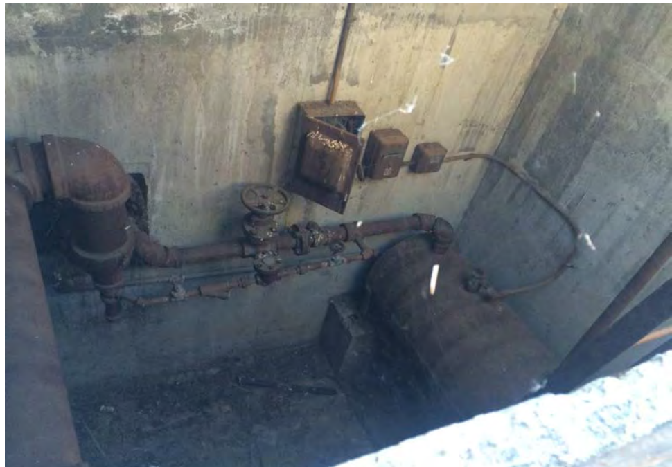
Photograph No. 12: View of the aboveground storage tank (AST located within the former Pump House basement enclosure.
