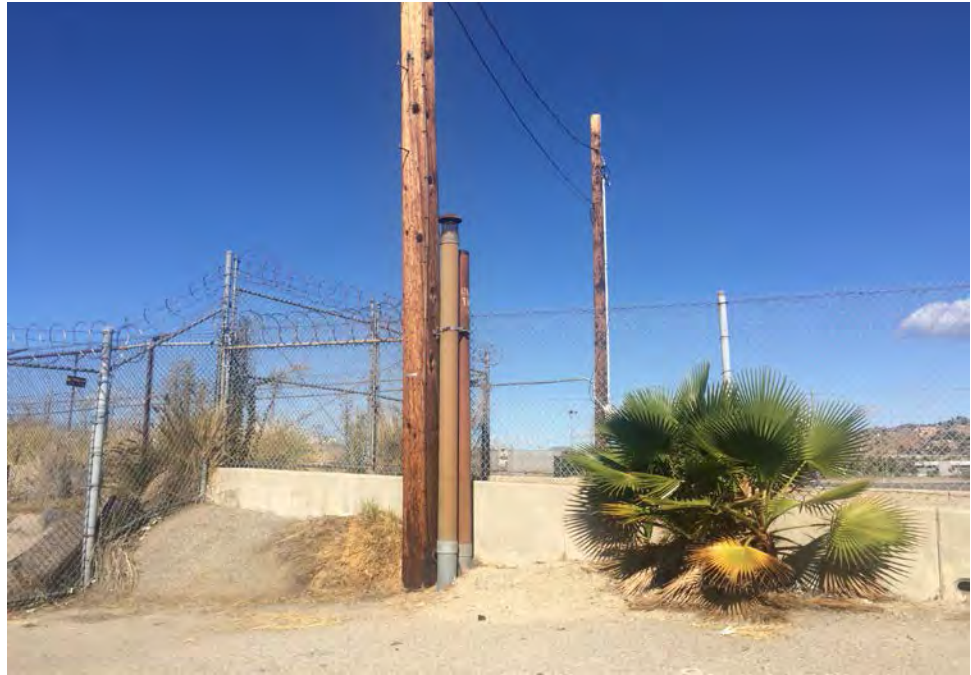
Photograph No. 13: View of vent pipe located on the central portion of the site, along an access road.
