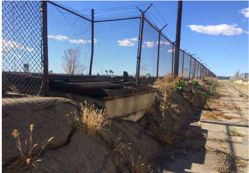
Photograph No. 11: View of the basement enclosure (aka former Pump House) located along an access road on the central portion of the site.
