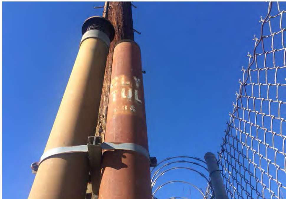
Photograph No. 14: Close-up view of vent pipe.
