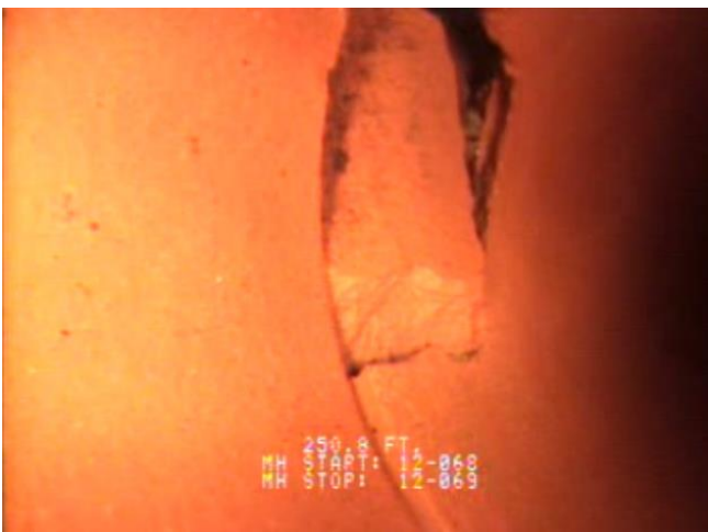
Broken pipe fragment
