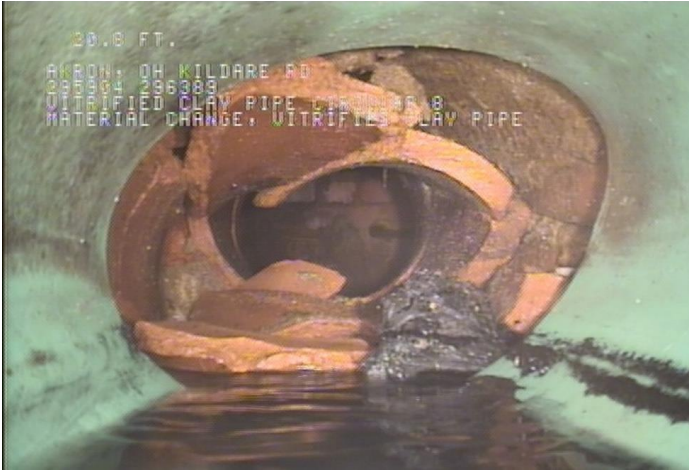
Lined portion of pipe deformed, unlined pipe beyond collapsed
