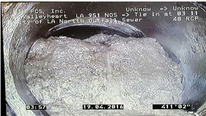
Blockage from roots and grease
