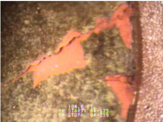
Minor crack in pipe at joint
