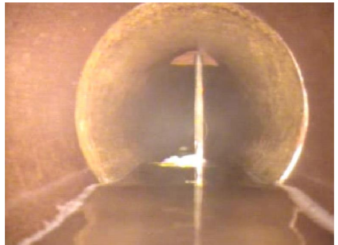
Grounding rod penetrating pipe, preventing maintenance efforts
