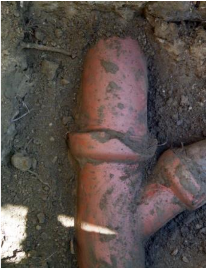
Chipped bell joint (exterior)
